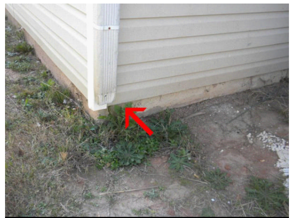
Elbow missing from downspout
