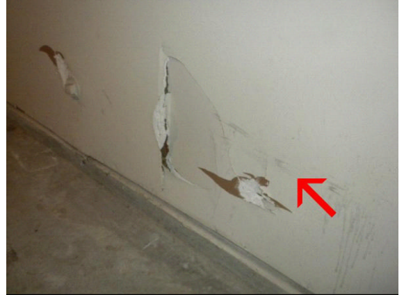
Damaged drywall in the garage
