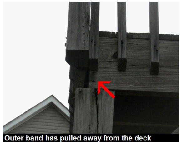
Outer band has pulled away from the deck
