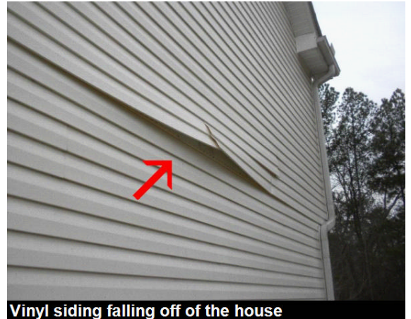
Vinyl siding falling off of the house
