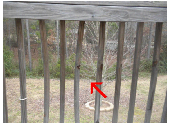
Warped railing pickets can be replaced
